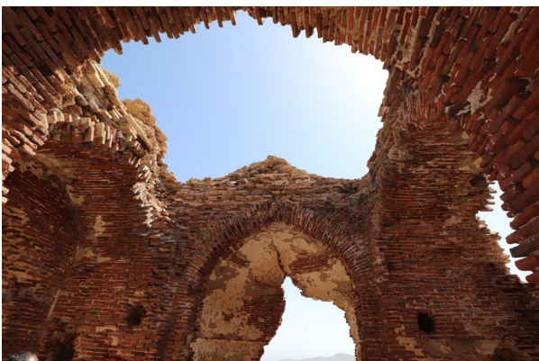
Fig. 6 - Surp Arakelots Church, detail of brick masonry from the walls and arches
