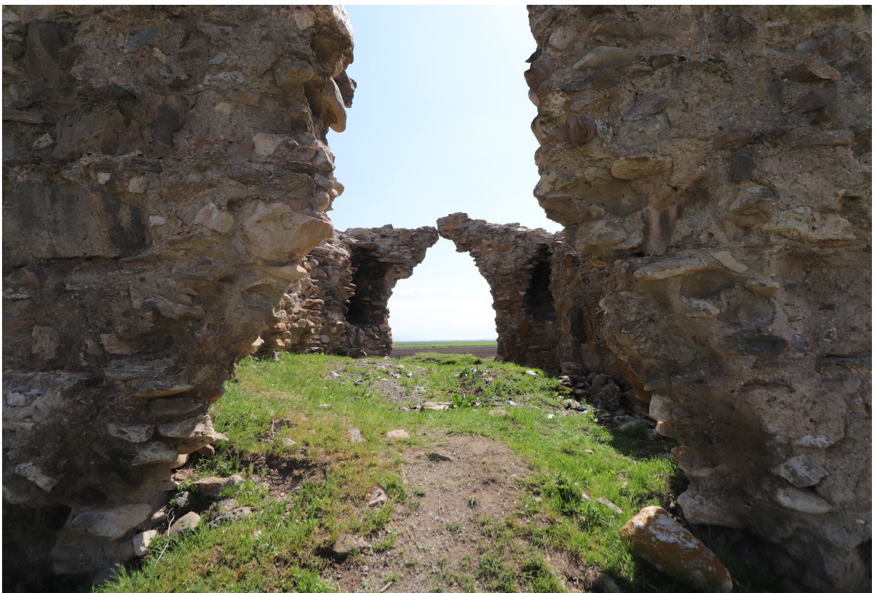
Fig. 2 - View of the interior from the western entrance, the collapsed western and eastern walls
