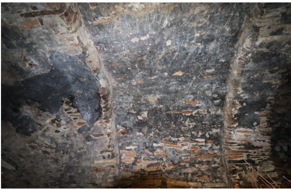
Fig. 4 - Interior walls, accumulation of soot
